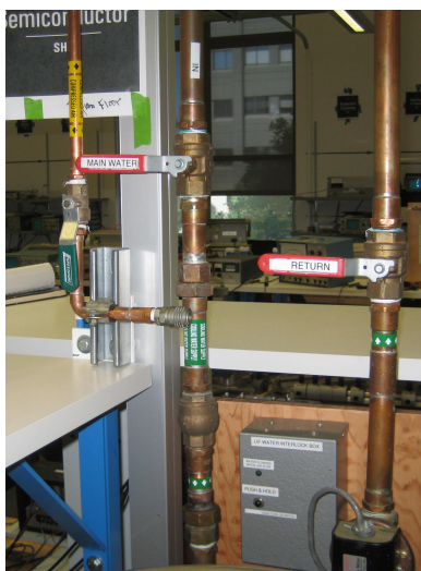
Figure 9: Water Control valves and interlock box Click here to see larger picture
