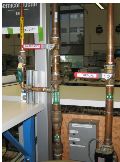
Figure 9: Water Control valves and interlock box Click here to see larger picture
