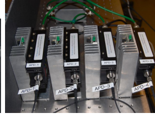
Figure 12: Fiber optic cables in to APDs
