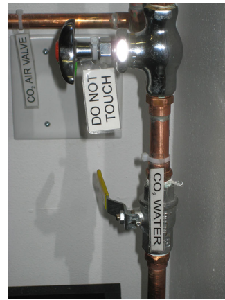
Figure 3: Water valve Click here to see larger picture
