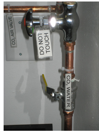
Figure 3: Water valve Click here to see larger picture
