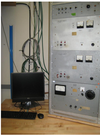
Figure 1: High Voltage Controls Click here to see larger picture
